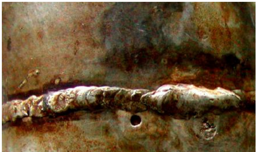
Example of pit corrosion caused by the presence of embedded iron
